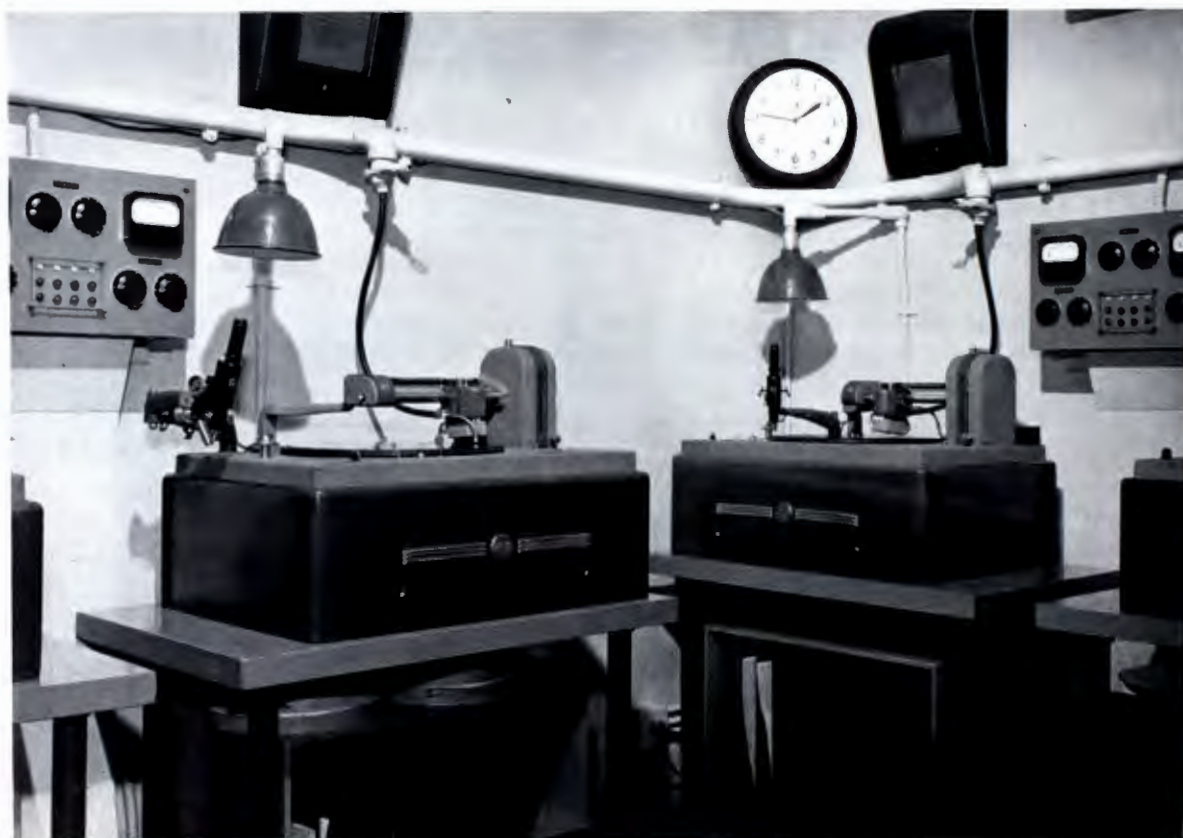
◆ An ideal recording installation at KECA, Los Angeles, Calif., showing two of the four RCA 73-B Professional Recorders. Note the conveniently located overhead lighting, the large size suction duct, and relatively short length of hose for chip removal.
